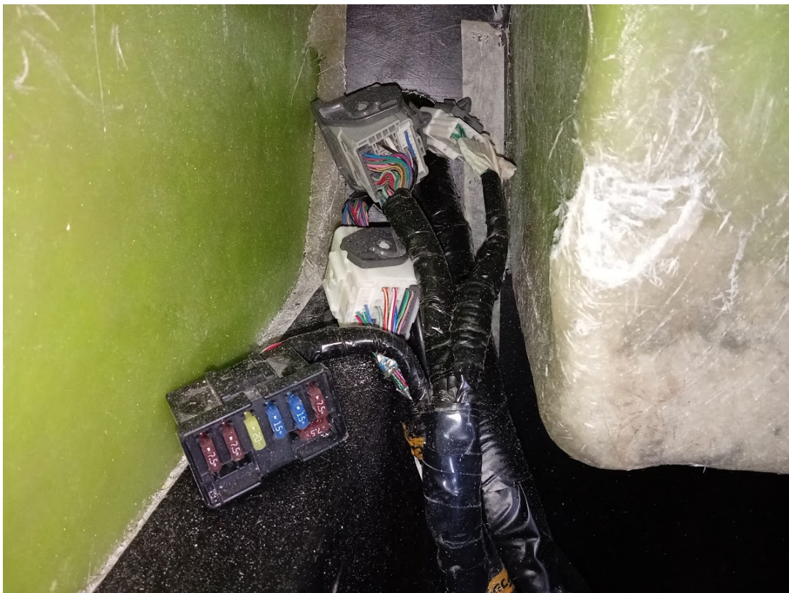
Couple up engine harness left side thru precut hole viewed from dashboard side
