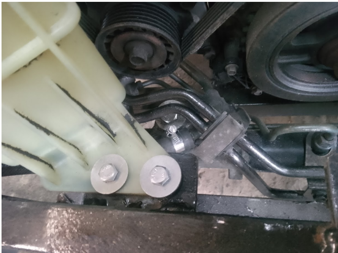
bolt power steering bottle 2 off M6 x 25 and couple up hydraulic hoses. Discard separate steel oil heat exchanger tube
